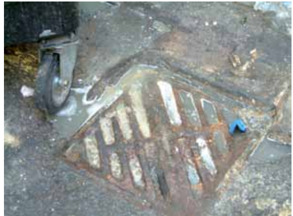
A surface water gully blocked with fat from a spillage
