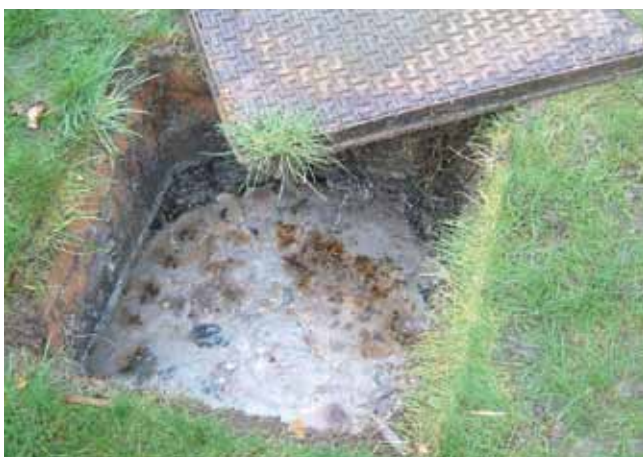
Fat building up in a manhole
