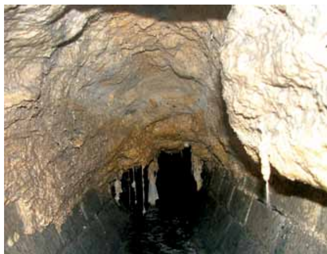
Fat beginning to block a sewer
