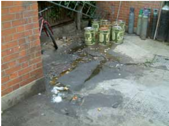
Avoid poor waste oil storage which could result in a sewer blockage or pollution incident
